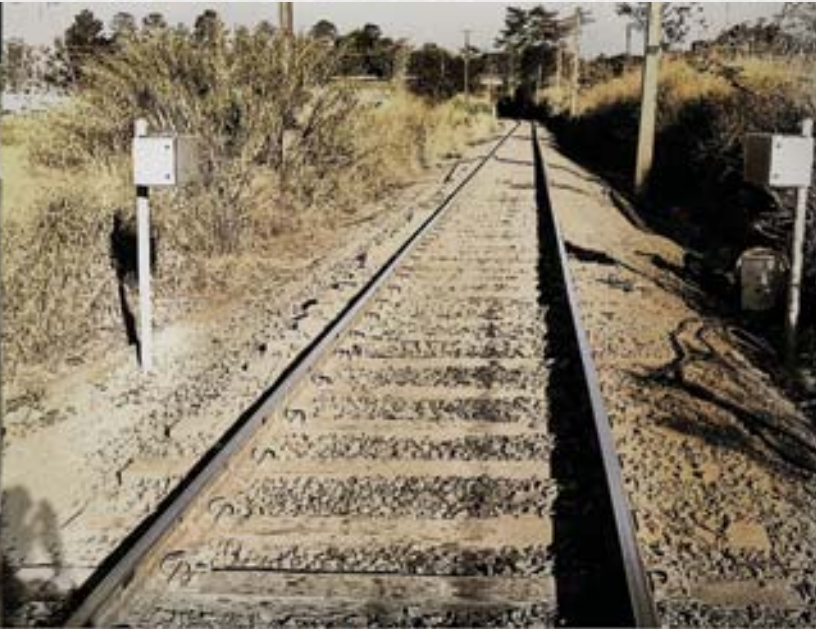
Antennas for tag reading, positioned beside the rails
